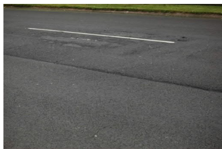
(c) "Suspect" Condition
