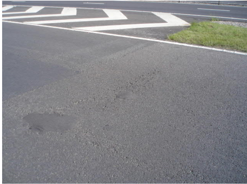
Figure 14: A5 Abbey Hill and Redmoor Surface Defects (Jones and Carswell, 2012)
