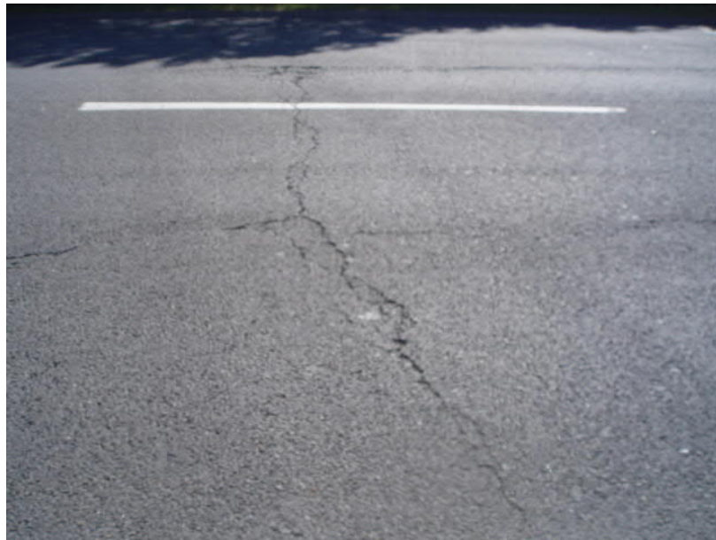
Figure 16 : A5 Abbey Hill and Redmoor with Potholing and Cracking (Jones and Carswell, 2012)
