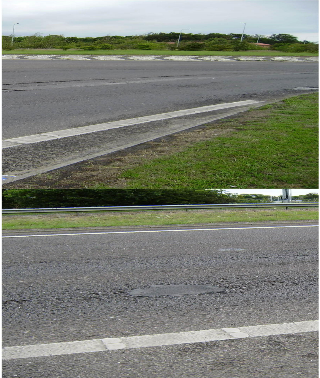
Figure 11: Fretting and Potholing on A12 N Station Road Roundabout (Jones and Carswell, 2012)
