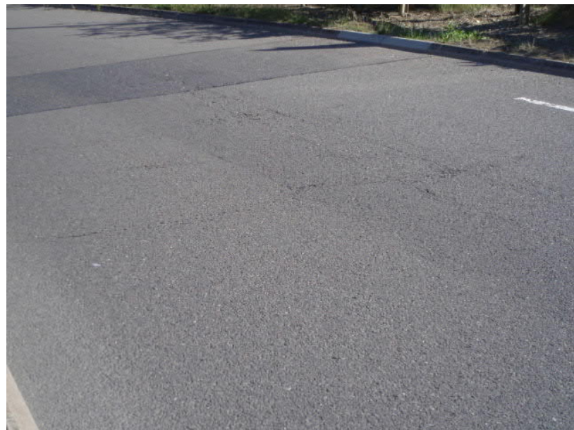
Figure 15: A5 Abbey Hill and Redmoor Surface Defects (Jones and Carswell, 2012)
